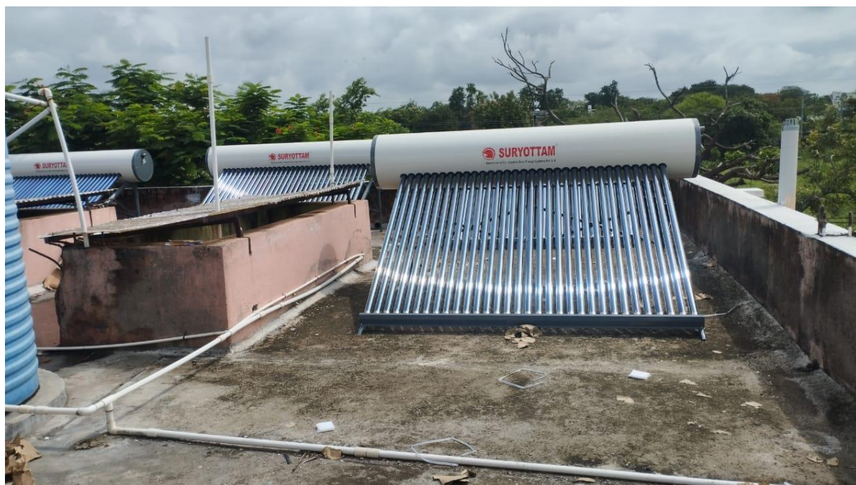
Solar water heating system at Hostel
